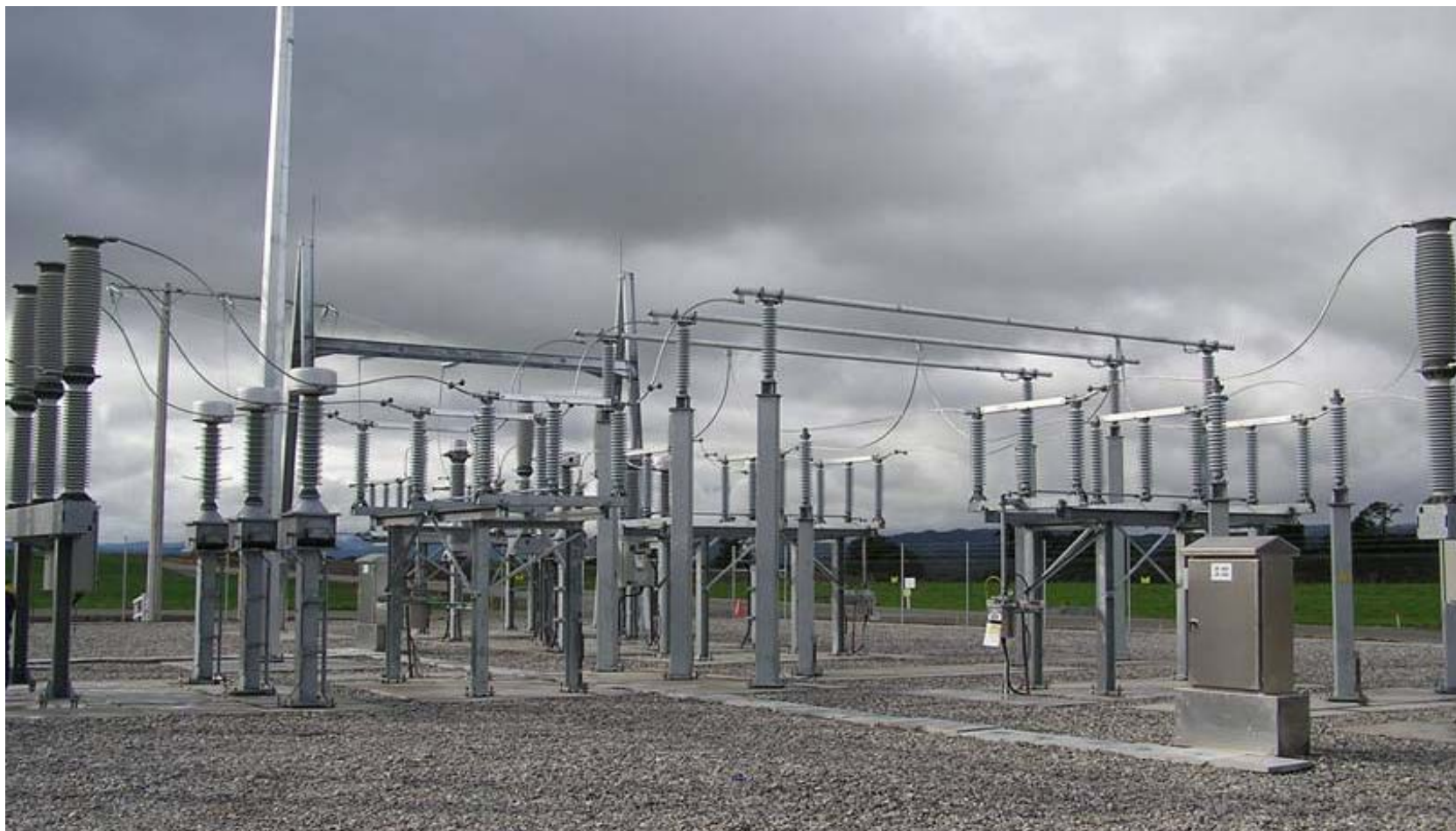
New Atarau substation
