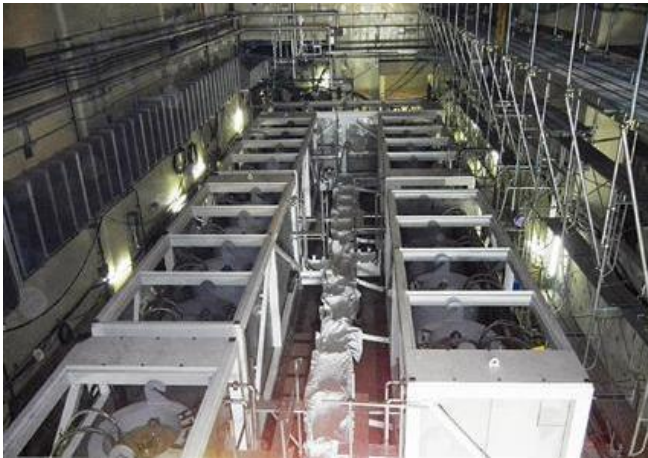
Contaminated Water Treatment System
